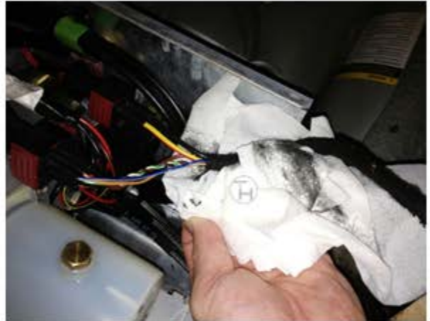
The friction tape wrapping the wire harness coming from the pump may be saturated with hydraulic fluid.
