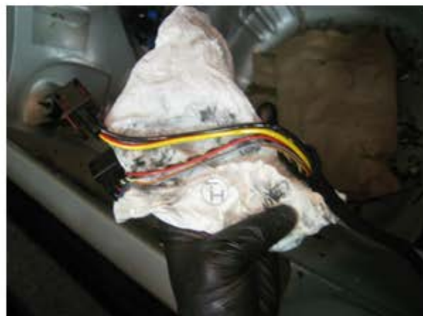
Carefully cut back the friction tape wrapping & clean the wires as much as possible.
